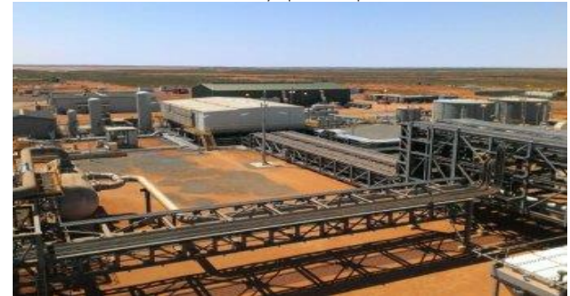
Macedon domestic gas plant, Onslow, WA
