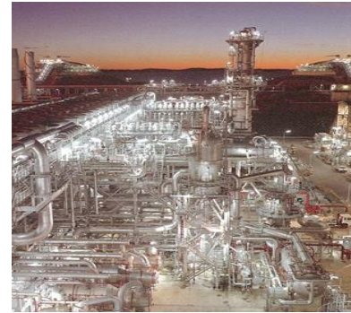
North West Shelf LNG plant at Karratha, WA
